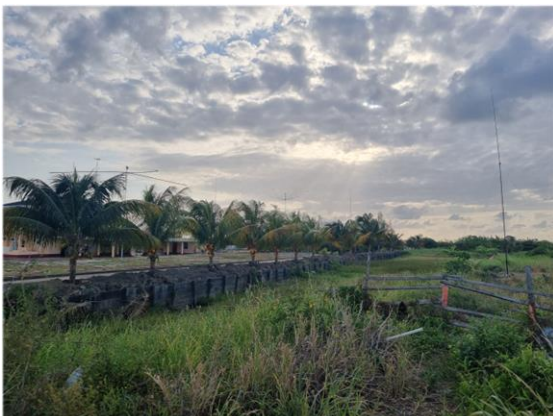
Various transmit antennas installed at the 8R7X Location.
